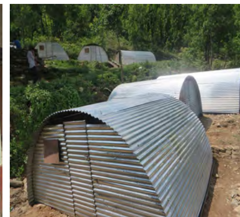
Where possible we give each family 14 metal sheets to build temporary shelter for the winter.
