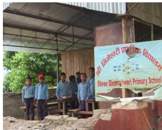
Only the roof of Ramechhap Primary School survived the earthquake. It is still in use as a temporary centre.
